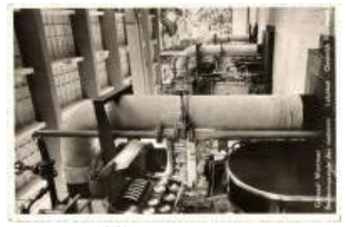
21818. ☒ Lelystad, Gemaa l Wortman / pumping st 1000
